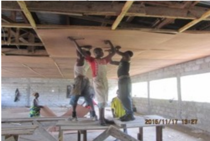
Preparing for the celebration, carpenters put up the ceiling in Castellanos Hall on the school campus. Labor and materials were purchased with donated funds.
